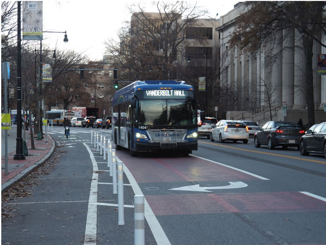
Photo taken from City of Cambridge Website. Installation of flexible posts on South Mass Ave in Cambridge.
