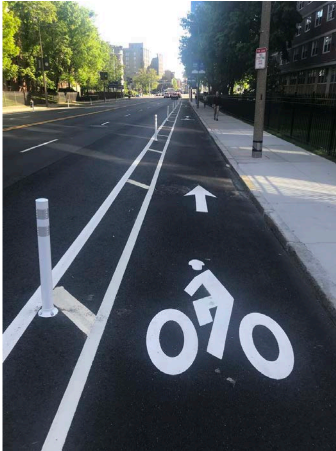
Photo of flexible posts installation on Brookline Ave in Boston. Photo Credit David Read of Farber/Harvard
