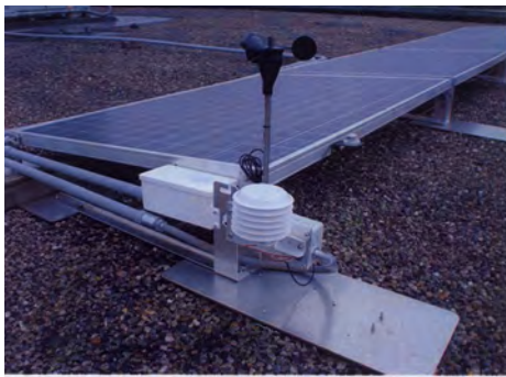
Photovoltaic Modules with a Heliostats Data Monitoring System installed at Worcester Polytechnic Institute.
