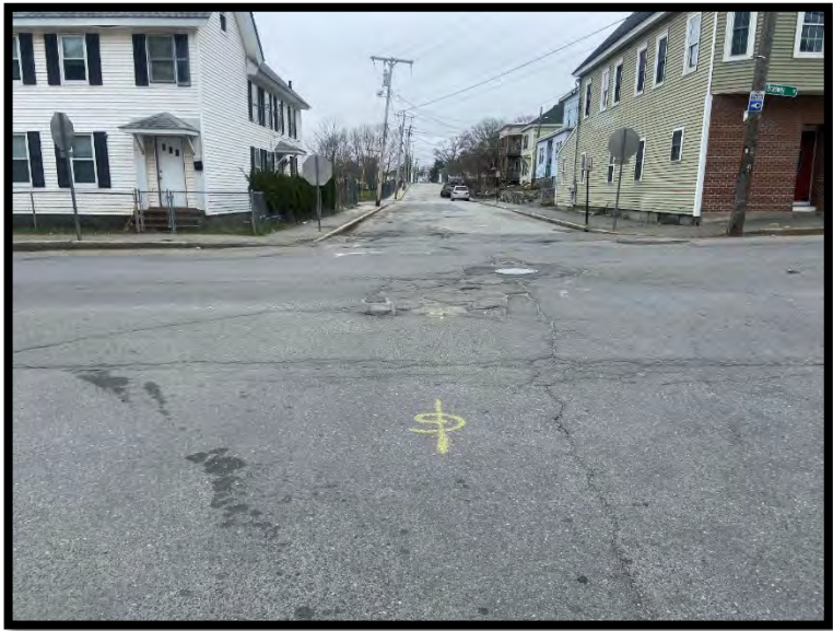
Example of street in need or rehabilitation (Walker St)
