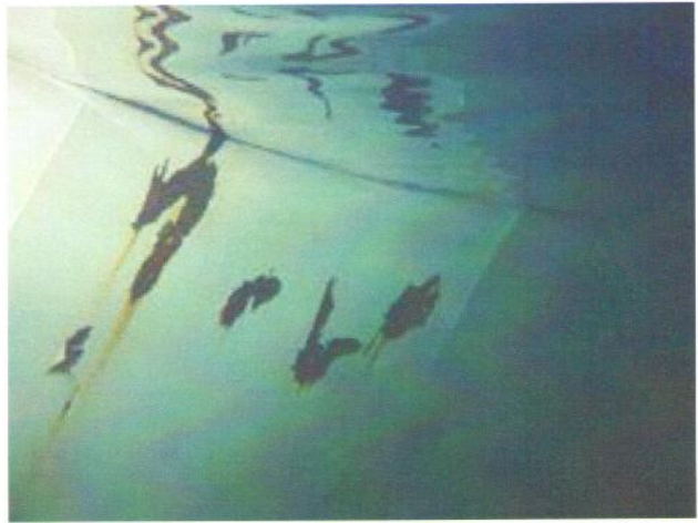
50 Interior Wall With Coating Loss, Exposed Underlying Steel, Mild Surface Corrosion And Mild To Moderate Staining
