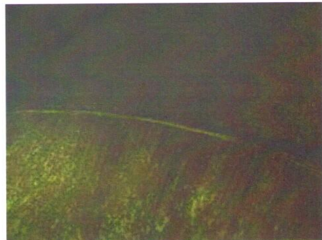
54 Interior Wall With Coating Loss, Exposed Underlying Steel, Mild Surface Corrosion And Mild To Moderate Staining
